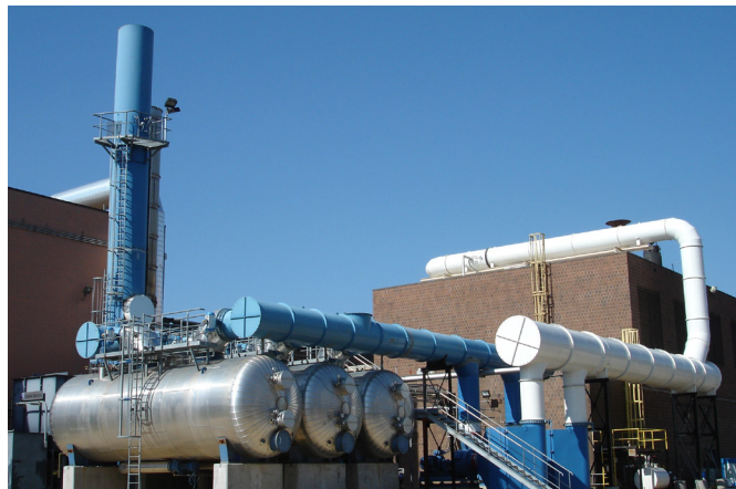
Activated carbon solvent recovery system
