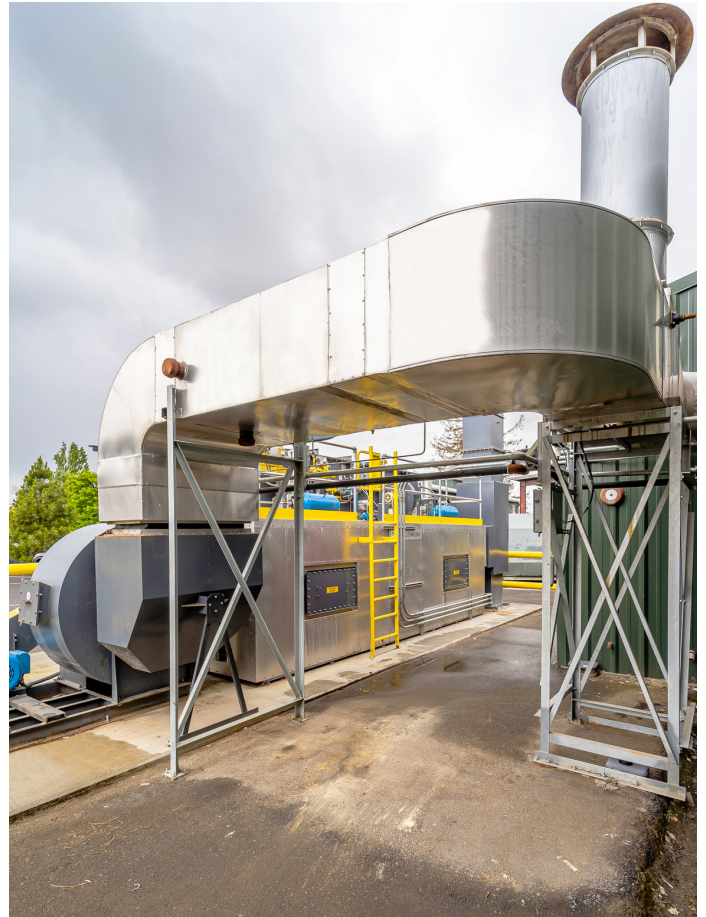
Oxi.X RM RTO abates formaldehyde generated by the asphalt shingle fiberglass mat manufacturing process.
